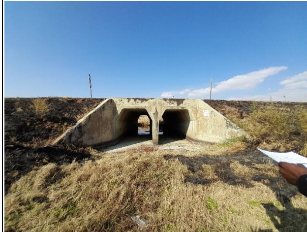
Culvert C1276 at km3.6 to be demolished and replaced with the same type of culvert.
