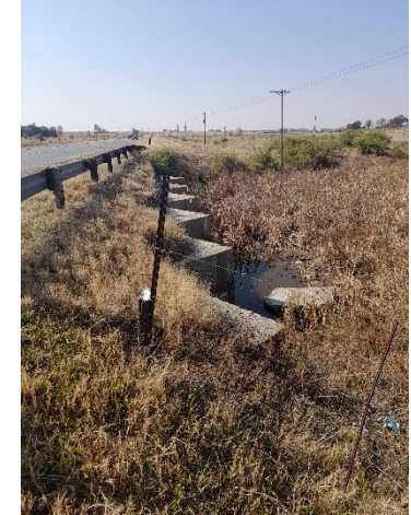
Culvert C002 at km7.4 to be extended on both sides. A tributary runs under the existing N14 at this point.
