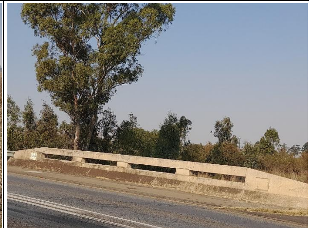
End of the N14-Section 12 road upgrade at km 58.4. R53 is under the N14.
