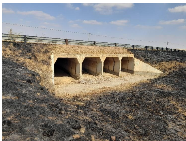
Culvert C4850 at km22.5 to be extended and widened on both sides.
