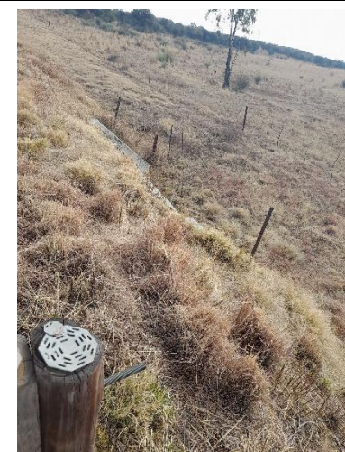
Box culvert C40 at km28.82 to be extended on both sides with two cells.
