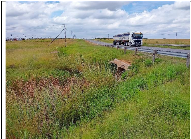
Culvert C34 at km52.2 to be widened and extended on both sides.
