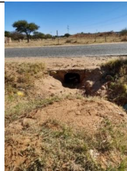
Existing culvert at Tabernacle School Intersection with N18 – Section 6 to be upgraded in situ.
