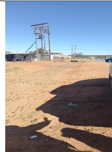
Storm water with culverts that are present near the N18 – Section 5. Intersection to be upgraded.
