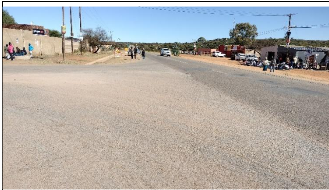
N18 – Section 5 - N18 and community access road to be upgraded at Km 40.277. No sensitive vegetation along the intersection. The area is transformed.
